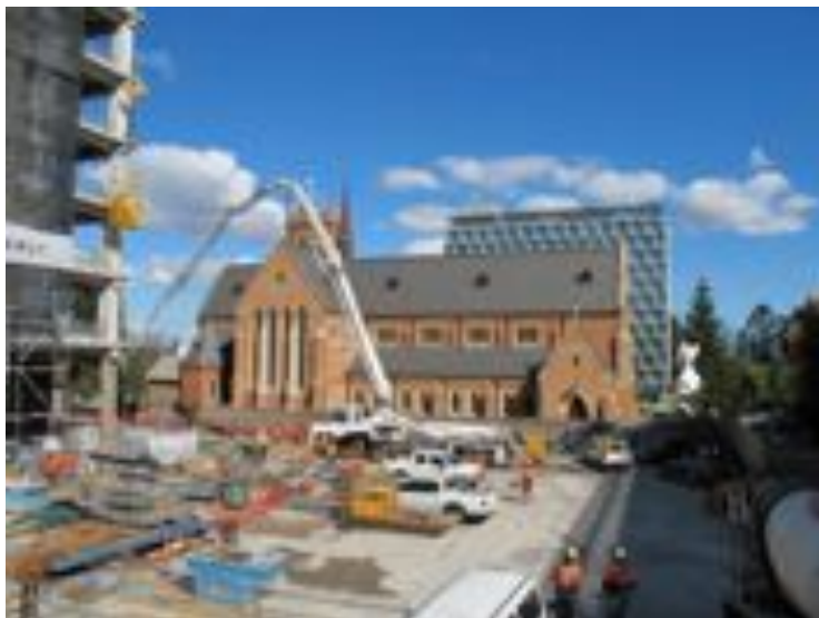
New library under construction. Pouring the ground floor slab. Photographer Cheryl Parrott, January 2013.
